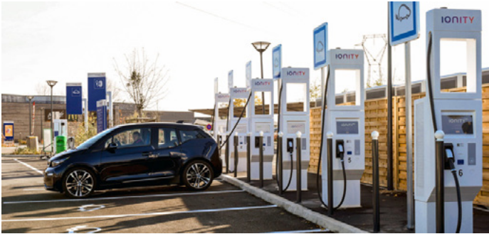
Figure 9: EV charging station on Vinci's French Autoroute Network, ASF
